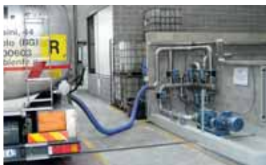
RECOVERY OILS PLANT
