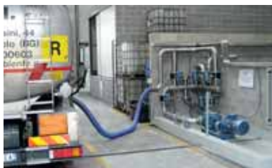
RECOVERY OILS PLANT
